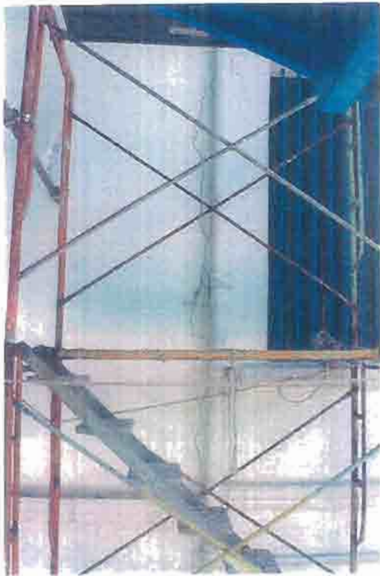
(E) Crack in exterior wall
