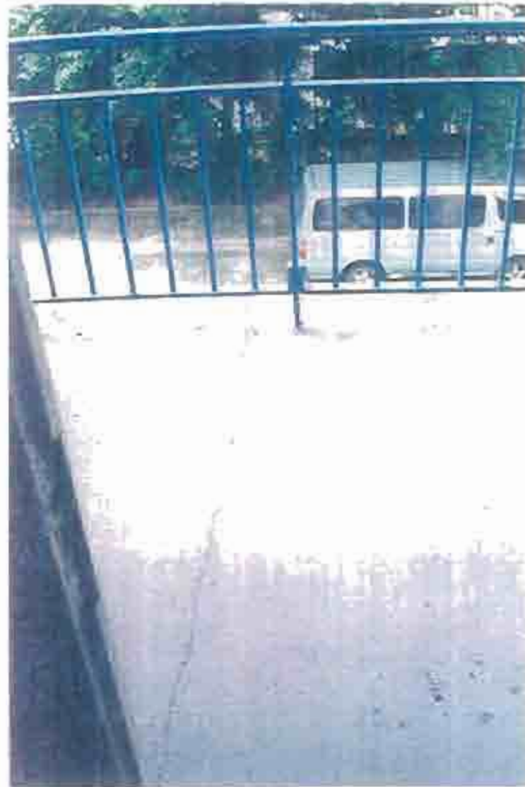
(F) Crack in concrete walkway
