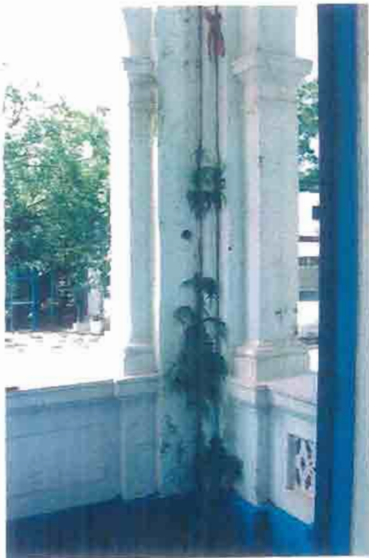
(A) Vegetation growth and water damage
