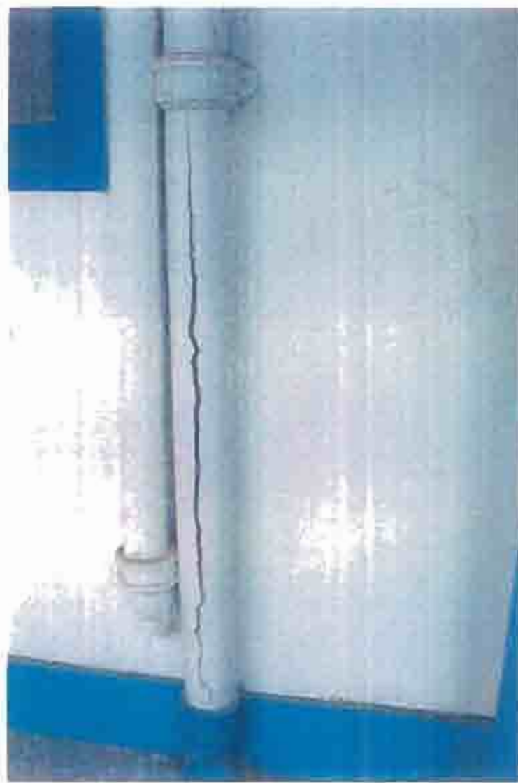
(B) Cracking in pipe
